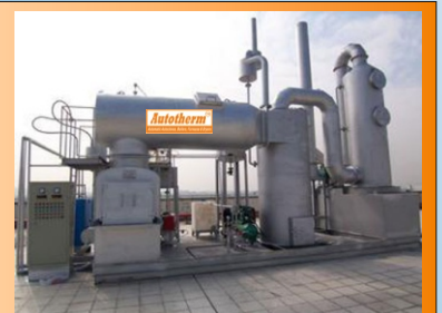
General/ Municipal Waste Incinerator
