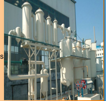
Pressure Treatment Plants, Steam Treatment Plant, Smell Treatment Plants, Bacterial/ Waste Treatment Plants
