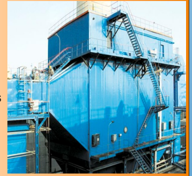
Electro Static Precipitator (ESP), Bag Filters & Cyclones, Heat Exchangers & Recuperators
